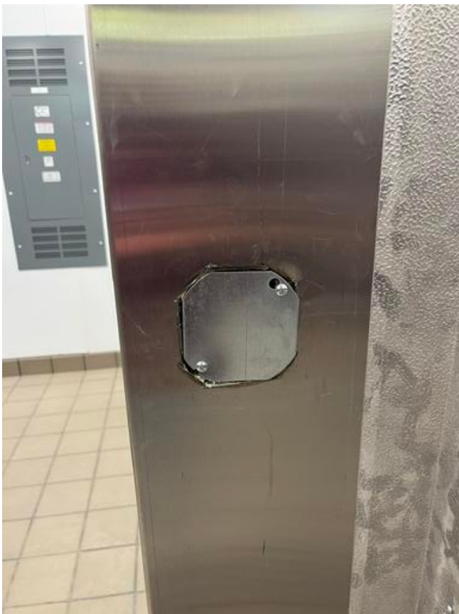
Missing Ansul Label
