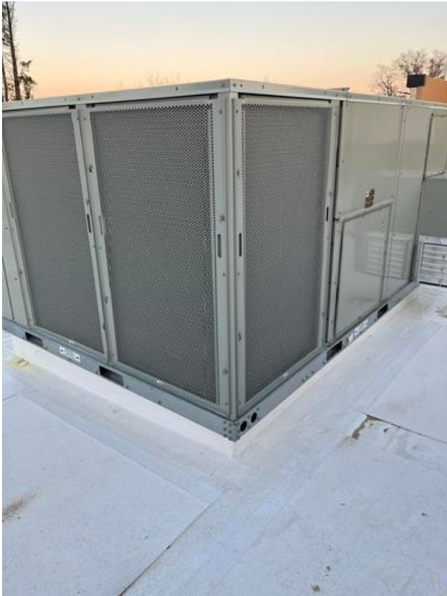
Missing Seismic Clips
