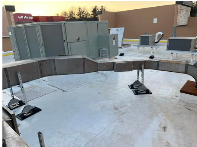
Grease Duct Supports
